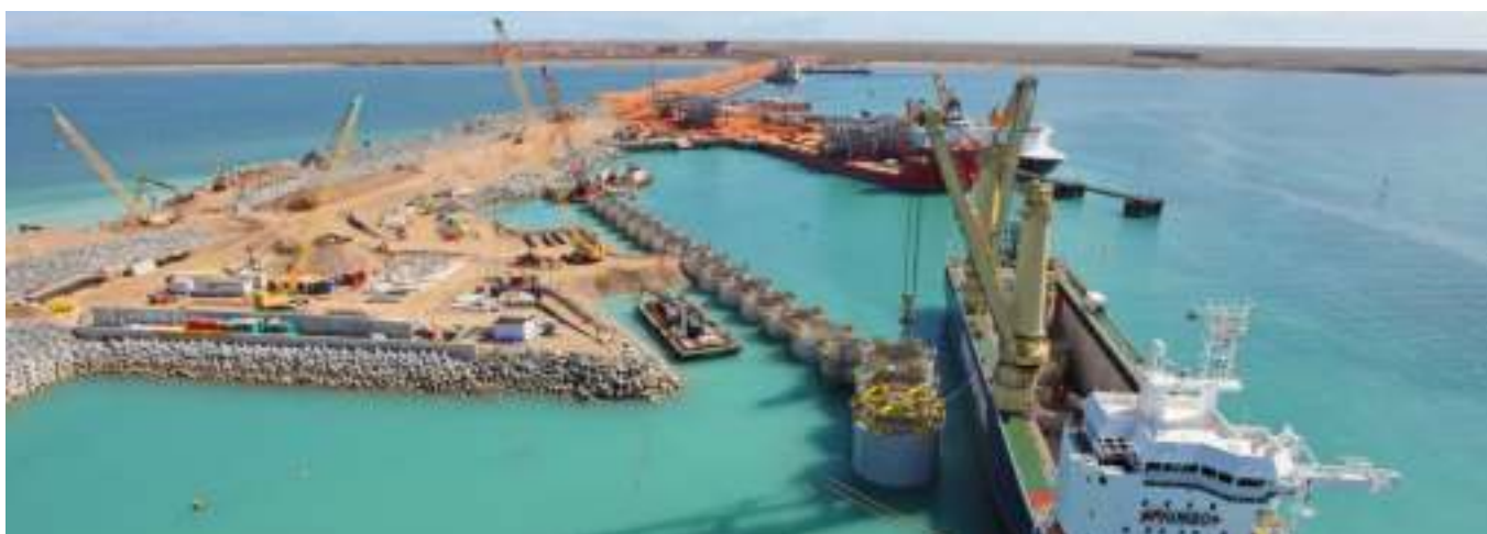
Construction works for the Gorgon project, Barrow Island, Western Australia. Photo: Jumbo, www.jumbomaritime.nl
